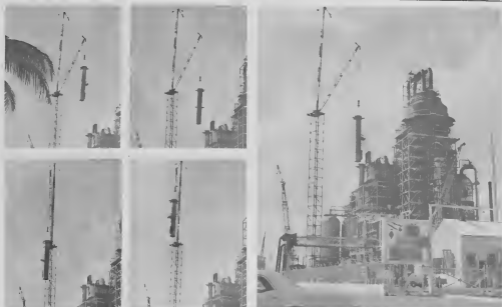
One major lift is handled by the 307-ft. derrick crane: a section of the PCAR smokestack. In about half an hour of skilled maneuvers, upward and downward, the section came down safely on the ground.
